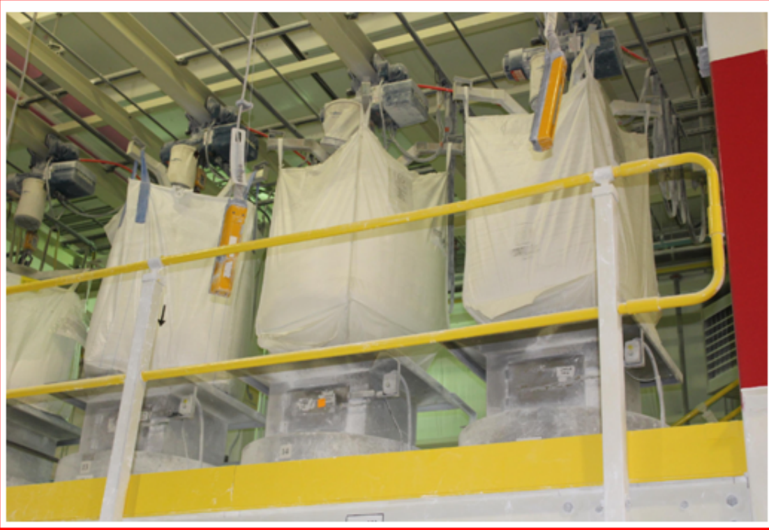
CHEMICAL FEED SYSTEM
