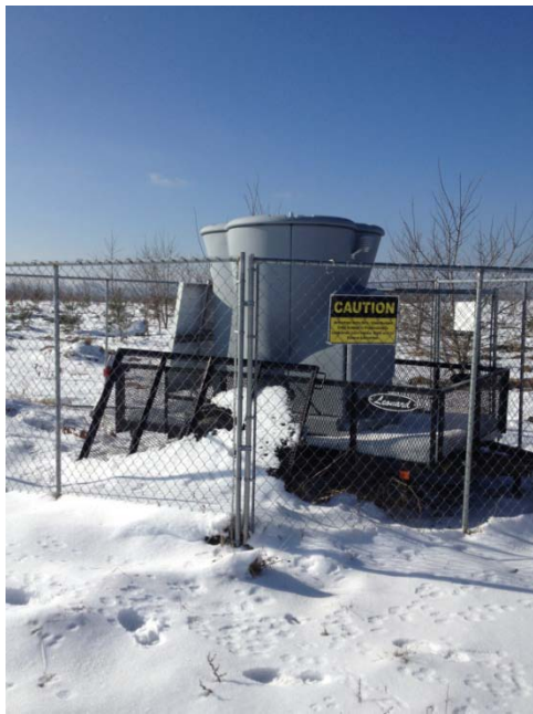
Bottom View: SODAR unit looking West prior to removal from site
