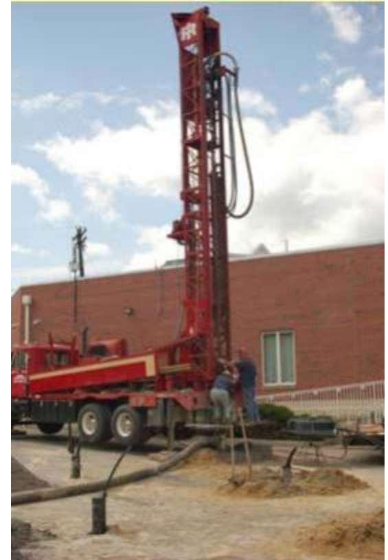
Buckhannon Geothermal Installation
